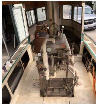
Boiler back-head looking forward
