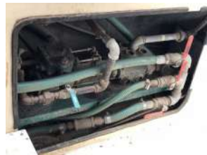
Worthington duplex steam pump: Can feed boiler, pump bilge, or spray water
