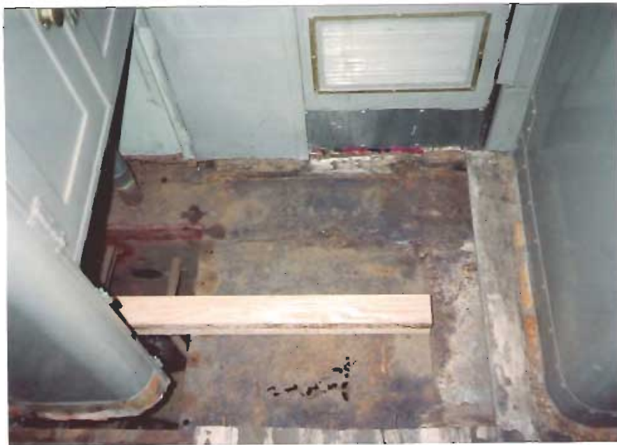
RUST OUT AT BRM C
